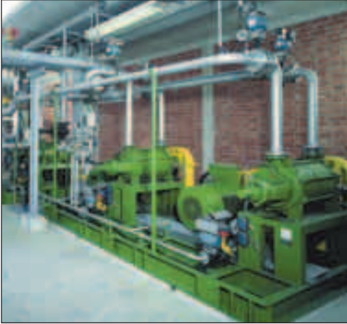
Fig 41: Liquid ring compressors installed in a drinking water treatment plant
